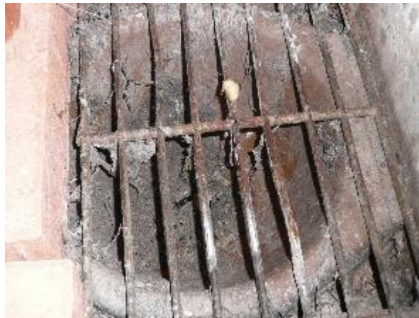
Eaves Gaping at eaves sheet joints Minor Defect Type: B Gapping at eaves sheet is further symptom of east side of building having moved away/subsided.
