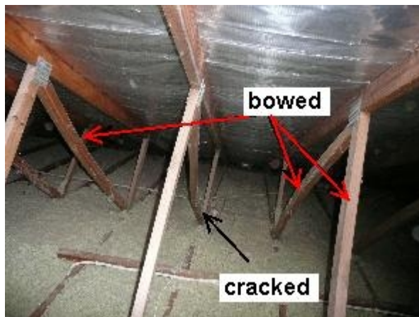
Roof framing Roof trusses show twist & excessive deflection Major Defect Type: B Truss joint failure has lead to trusses distorting & twisting and to cracking of some truss webs.
